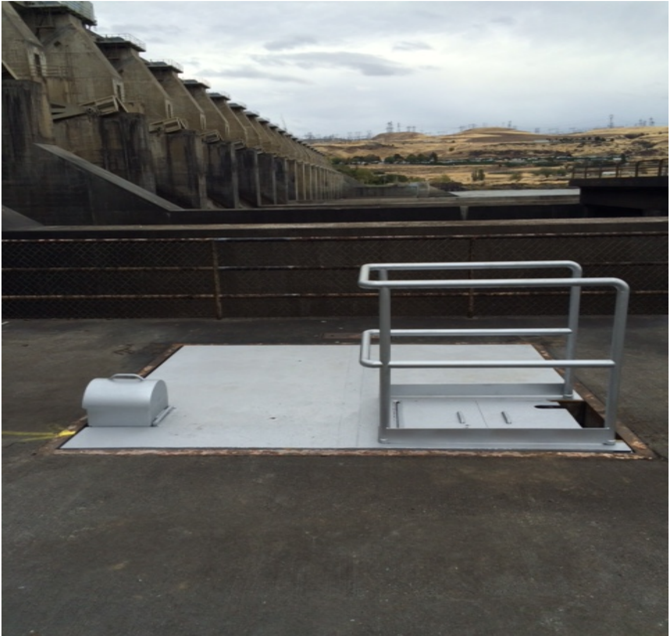
New north fishway dewatering pump motor with protective access hatch
